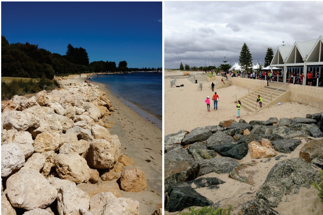
Sea walls are an example of hard active interim protection measures. Designed well, they can integrate well into the development of beach amenities, although they can exacerbate erosion (beach loss) in front of the wall over time if ongoing sand nourishment is not undertaken.
