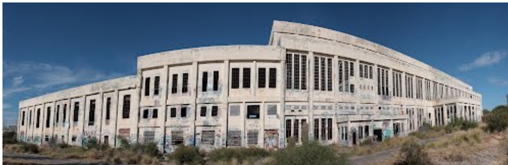
Fig.1: West Elevation of Power Station to a usable recreational beach and Cockburn Sound.
